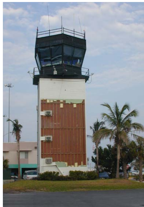
Damage to Key West International Airport's control tower after Hurricane Wilma
